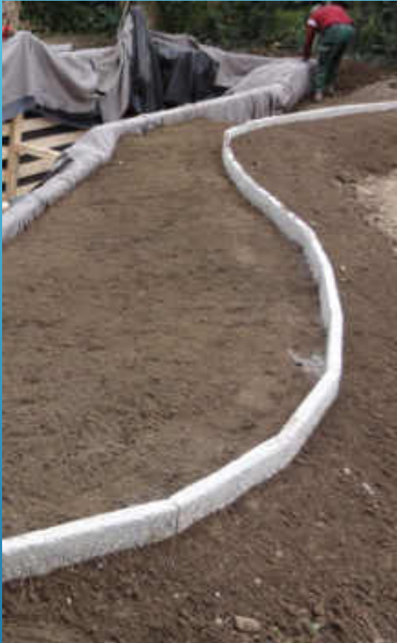
Betonrandleisten Concrete skirting boards
